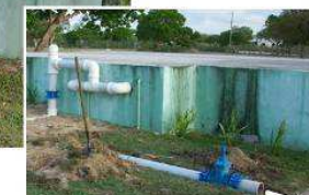
first-flush diverter and valve
